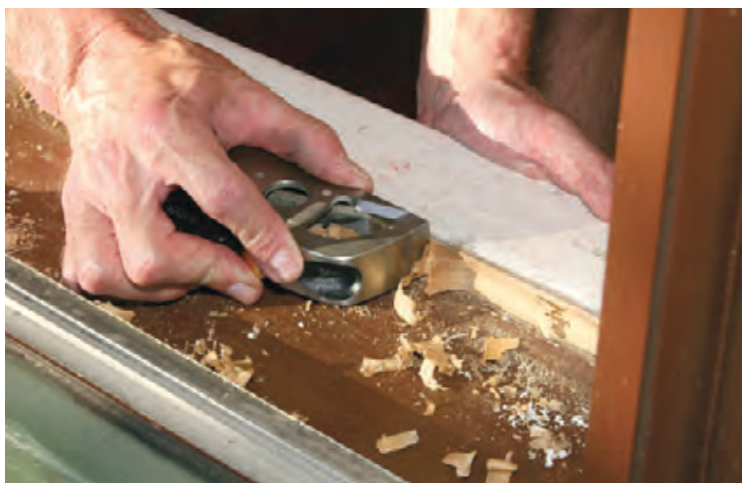
Figure 5. Before the weatherstripped sash can be reinstalled, the stool must be scribed and trimmed to allow for the thickness of the brush seals on the face of the side rails. A \frac{1}{16} -inch-wide gap, scribed with a carpenter's pencil, allows for expansion (top). A bullnose plane with a removable toe piece cuts away the excess stock with a minimum of dust (above).
